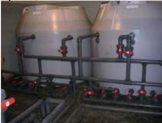
White Spruce's 7,500 gallons per day Water Treatment Plant
