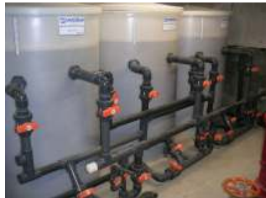
Echo Valley's 2,000 gallons per day Water Treatment Plant
