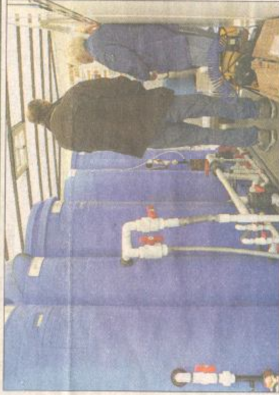
Residents of the Town of Manitou and the R.M. of Pembina were invited to an open house at the water treatment plant last week, and had the opportunity to see a "BioFiltration" water treatment demonstration inside this portable trailer mounted unit.
