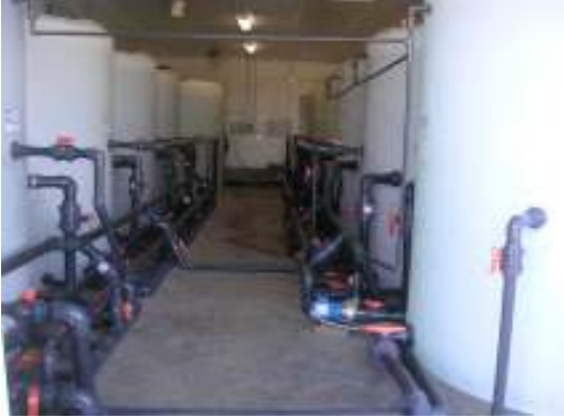
Manor's 50,000 gallon per day Water Treatment Plant
