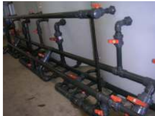
Manor's 50,000 gallon per day Water Treatment Plant
