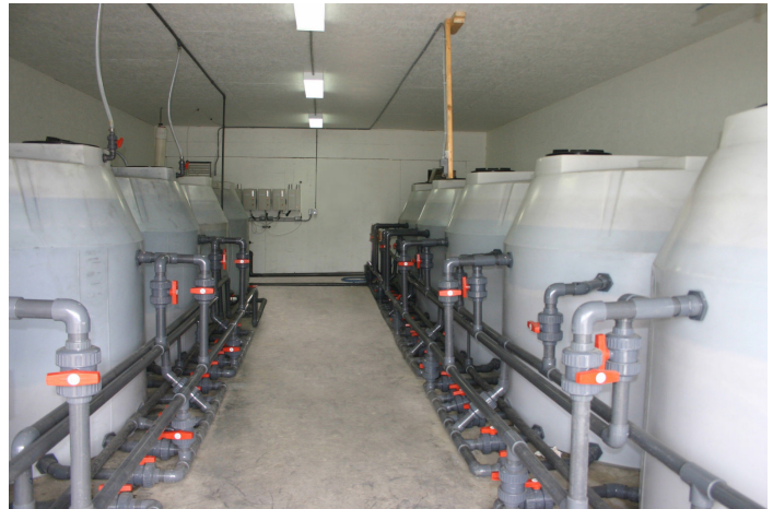
The new Mainstream BioClear 22000 SCOR (Sand, Ozone, Roughing, Carbon) Water Treatment Plant
