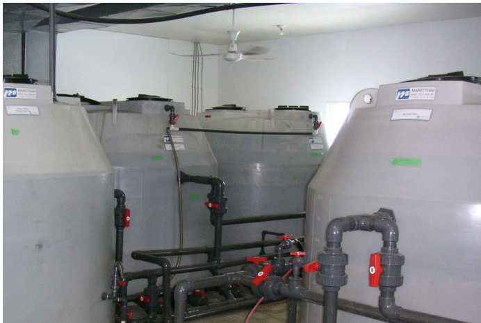
The new Mainstream BioClear 10000 SCOR (Sand, Ozone, Roughing, Carbon) Water Treatment Plant
